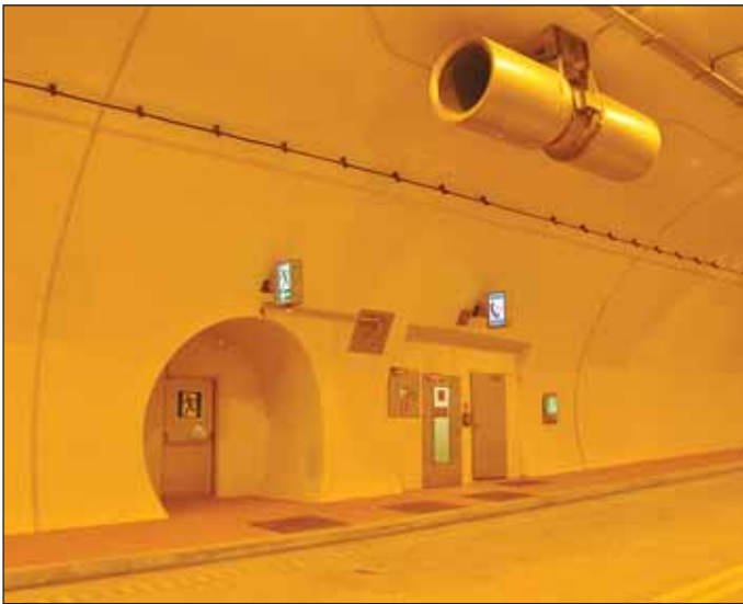
Obr. 8 Pohľad na hotové sekundárne ostenie tunela Fig. 8 View of the completed secondary tunnel lining
